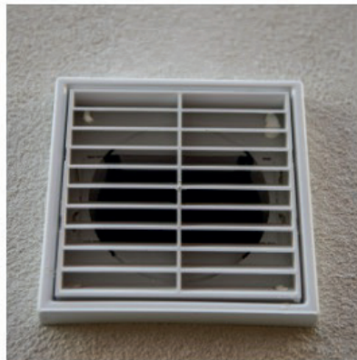
Bentley and Scott's ventilation system ADRIAN SHERRAT FOR THE SUNDAY TIMES
