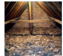
Loft insulation Extra layers of insulation (up to 300mm) are rolled out between and over the joists in the loft space.
