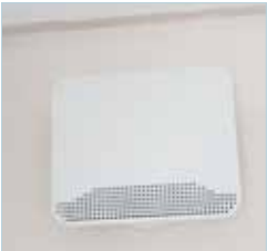
Ventilation. Good ventilation and moisture extraction is very important in high occupancy houses.
